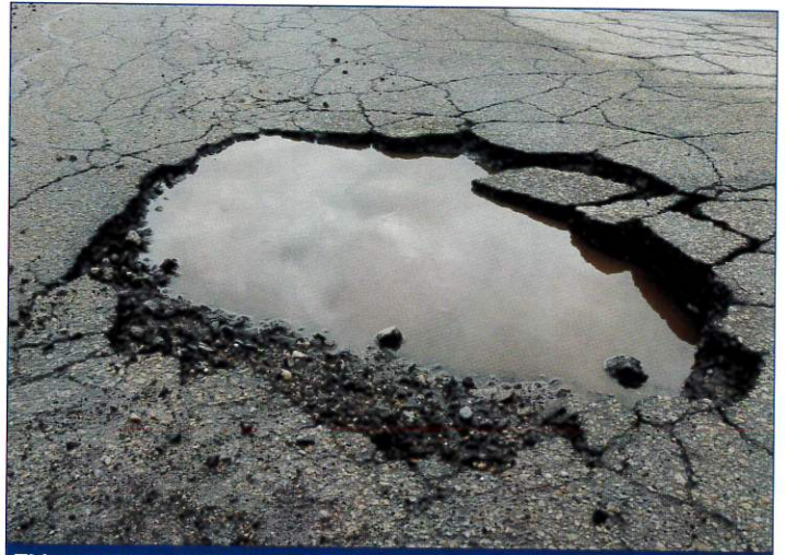
This can damage your car. See it - report it.
